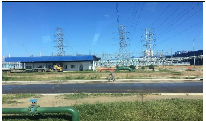
Fig 04. 110KV Electric Grid
